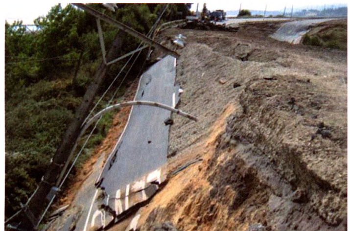
Figure 15: Road embankment collapse at the entrance of the town of Lota
