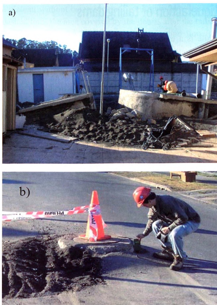
Figure 8: a) Uplift of buried sewage tanks in San Pedro del Valle and b) manhole uplifted
