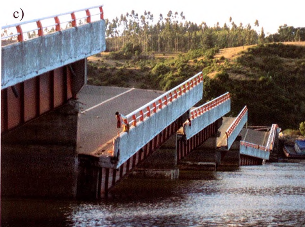
Figure 14: Tubul Bridge a) aerial view showing complete bridge collapse, b) failure of bridge access and c) decks fallen down
